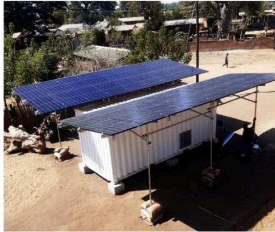
Figure 14 Dedza Microgrid in Malawi
